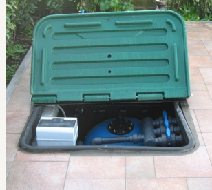
Underground plant room.
