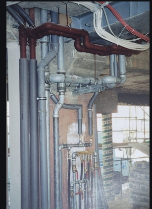
Risers and technical networks.
