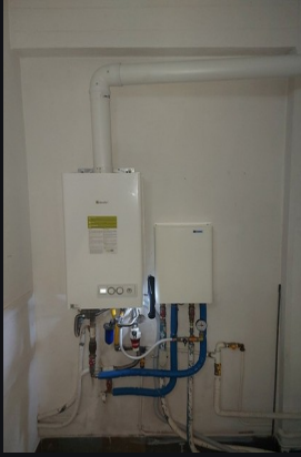
Boiler and hydronic circuit.
