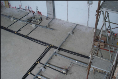
Water/sanitary systems and drainage for technical areas, refrigerated counters and fish departments.
