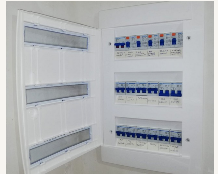
Completed electrical switchboard.
