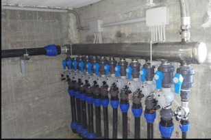
Water distribution and manifolds.
