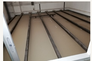
Suspended-ceiling framework and metalwork.
