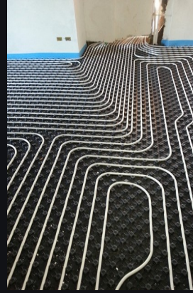
Radiant floor heating.
